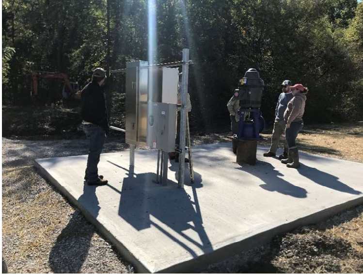
Figure 8 – Recently Constructed Water Supply Well
