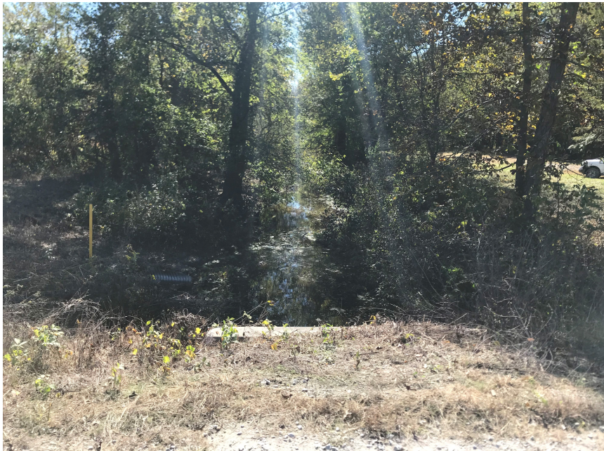
Figure 7 - Existing Channel, Undersized and Overgrown with Vegetation & Trees
